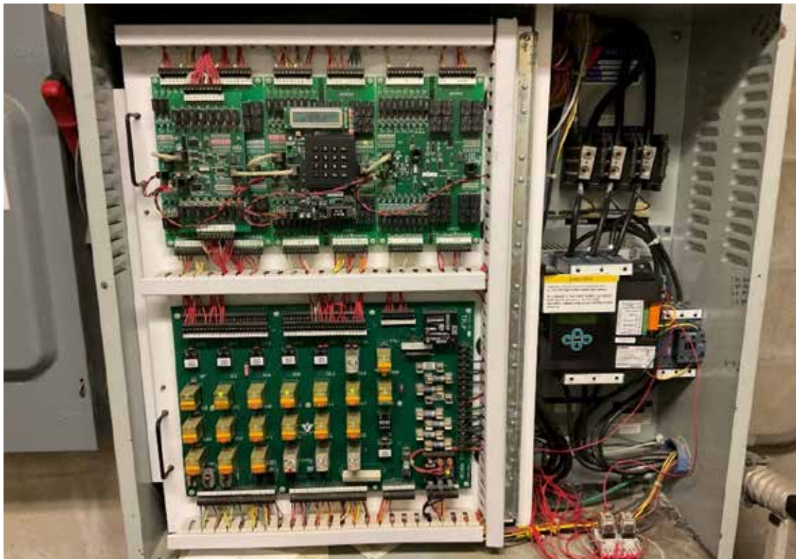
Bldg 100 - Elevator Equipment
