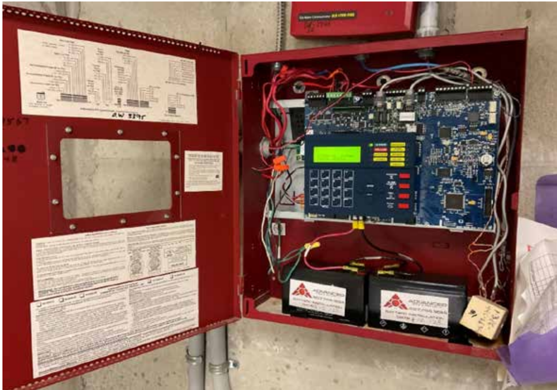
Bldg 100 - Fire Alarm Panel
