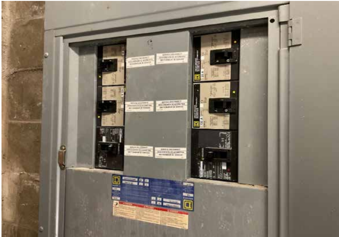
Bldg 300 - Electrical Breakers
