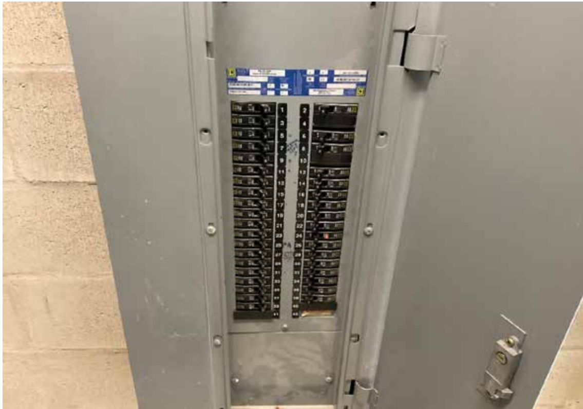
Bldg 100 - Electrical Breakers
