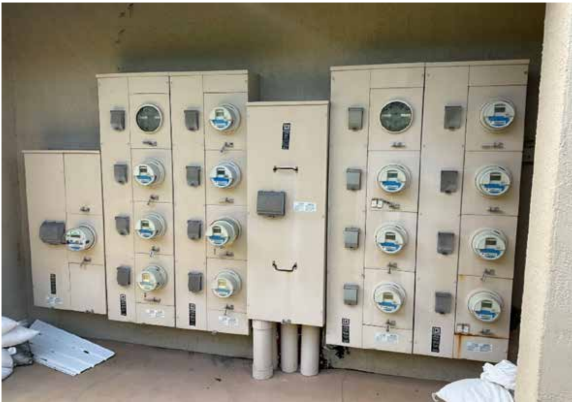
Bldg 300 - Electrical Panel/Meters
