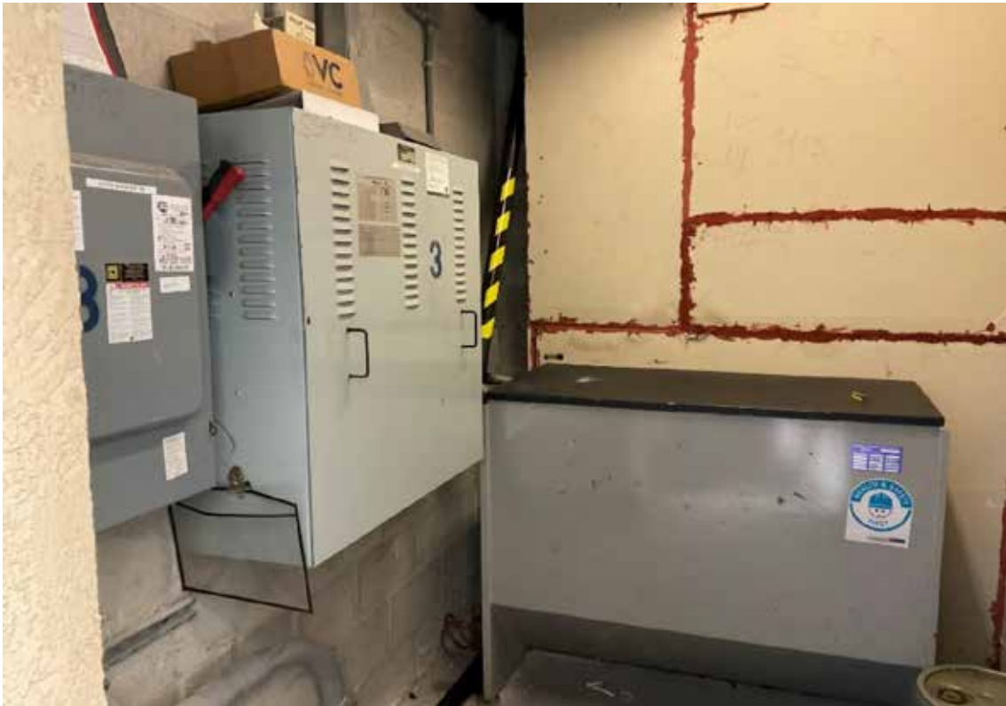
Bldg 300 - Elevator Equipment
