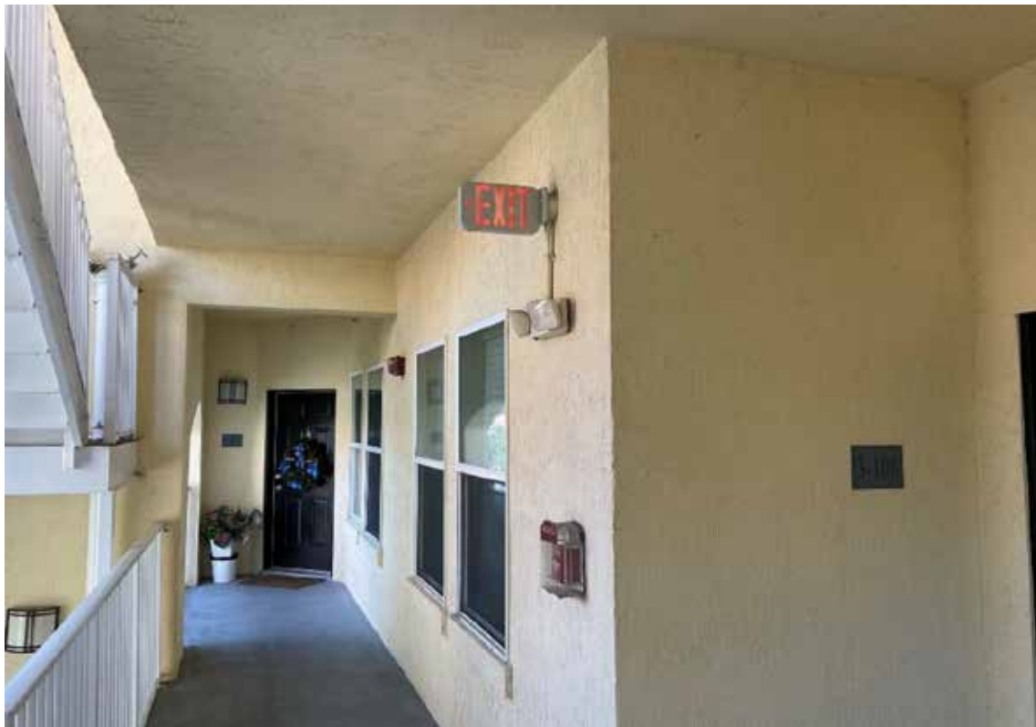
Bldg 300 - Fire System
