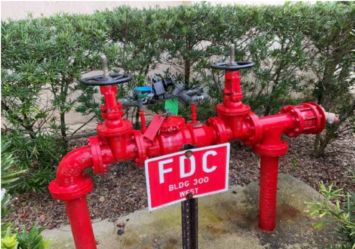
Bldg 300 - Backflow Preventer
