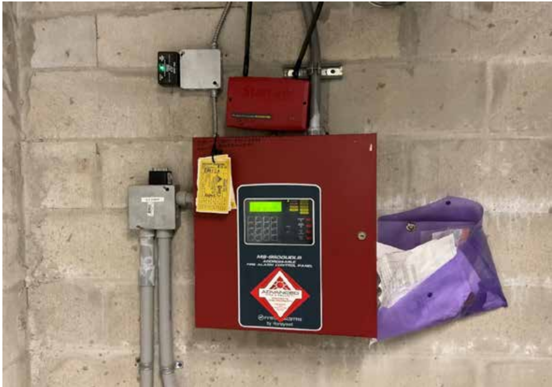
Bldg 100 - Fire Alarm Panel
