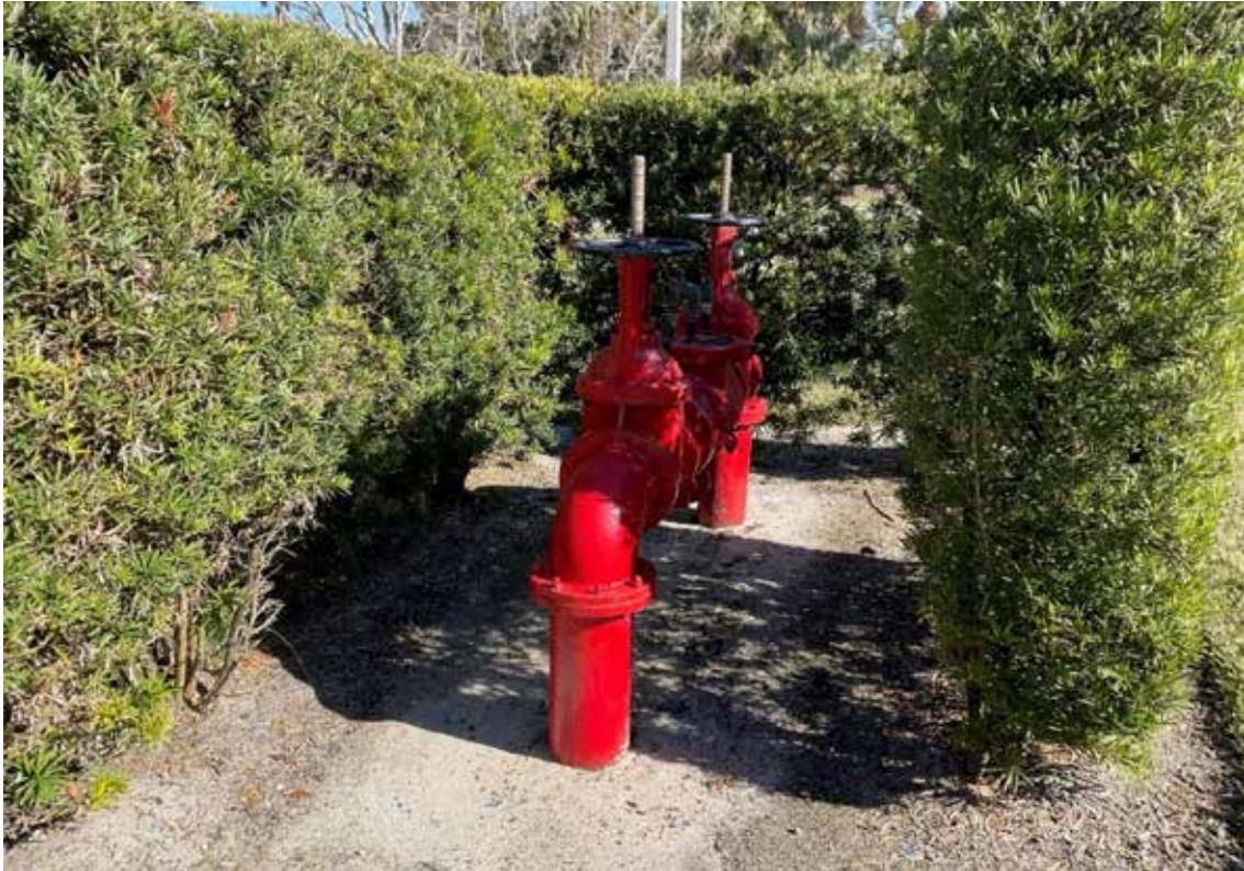
Backflow - Property Fire Systems
