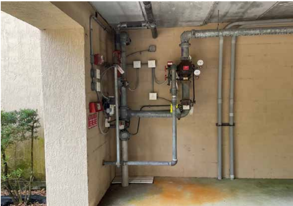
Bldg 300 - Dry Fire System
