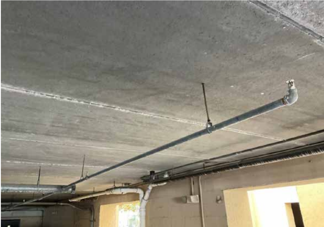
Bldg 100 - Fire Sprinklers
