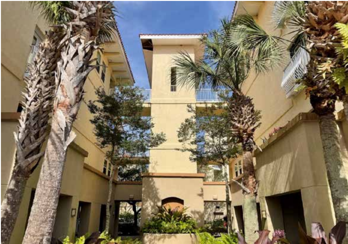
Bldg 300 - Missing Soffit
