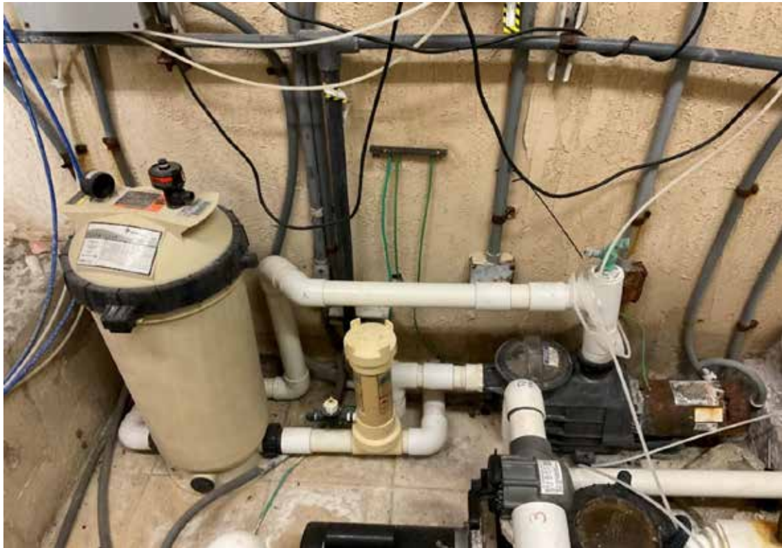
Water Feature Equipment
