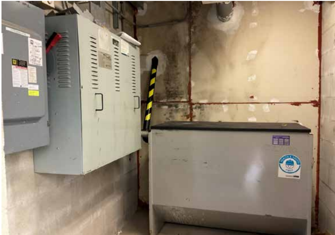
Bldg 100 - Elevator Equipment
