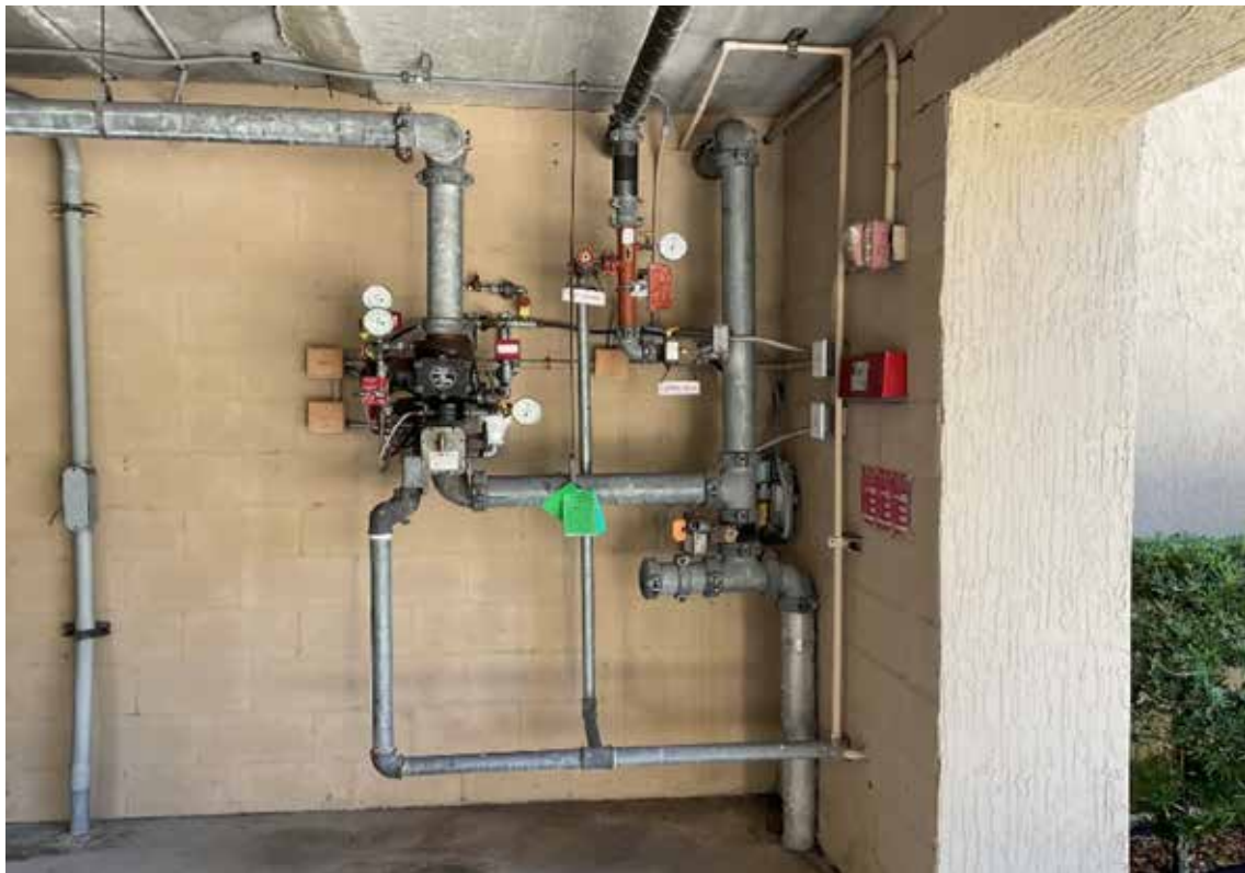
Bldg 200 - Dry Fire System
