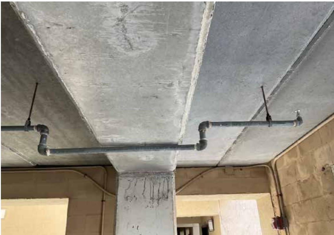
Bldg 300 - Fire Sprinklers
