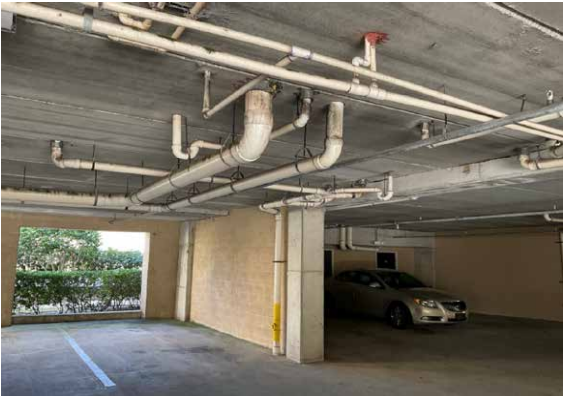
Bldg 200 - Plumbing Lines
