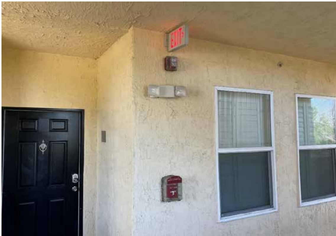
Bldg 100 - Fire System
