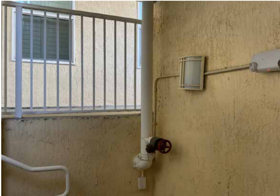
Bldg 100 - Fire Standpipe
