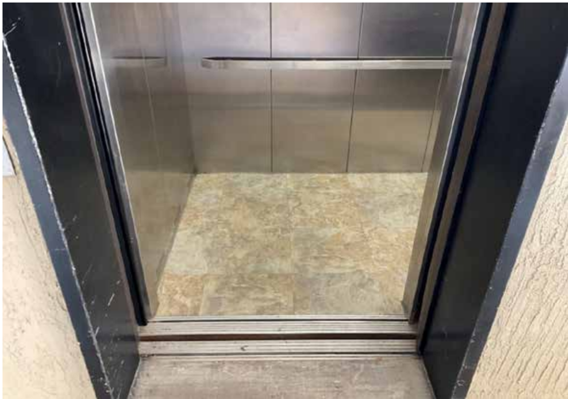
Bldg 300 - Elevator Cab
