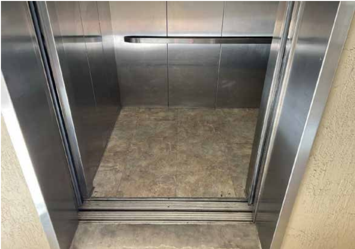
Bldg 200 - Elevator Cab
