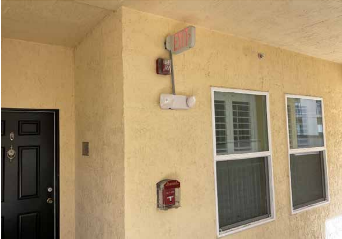
Bldg 200 - Fire System
