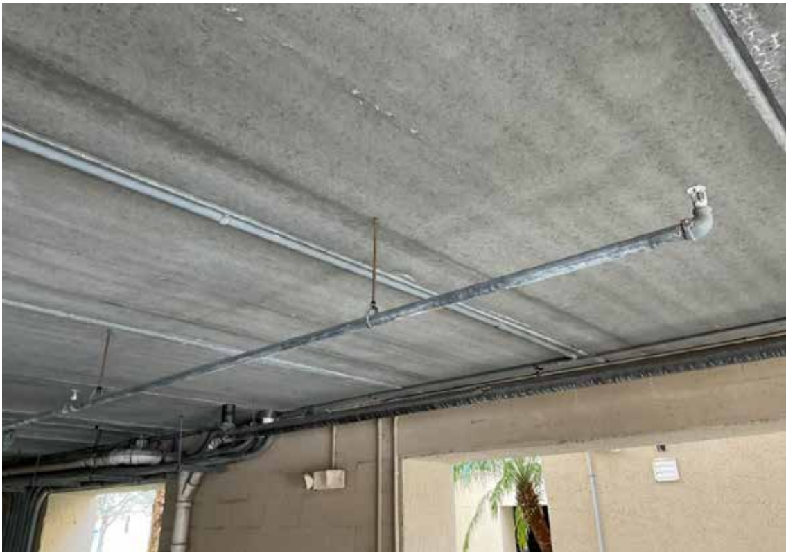
Bldg 200 - Fire Sprinklers
