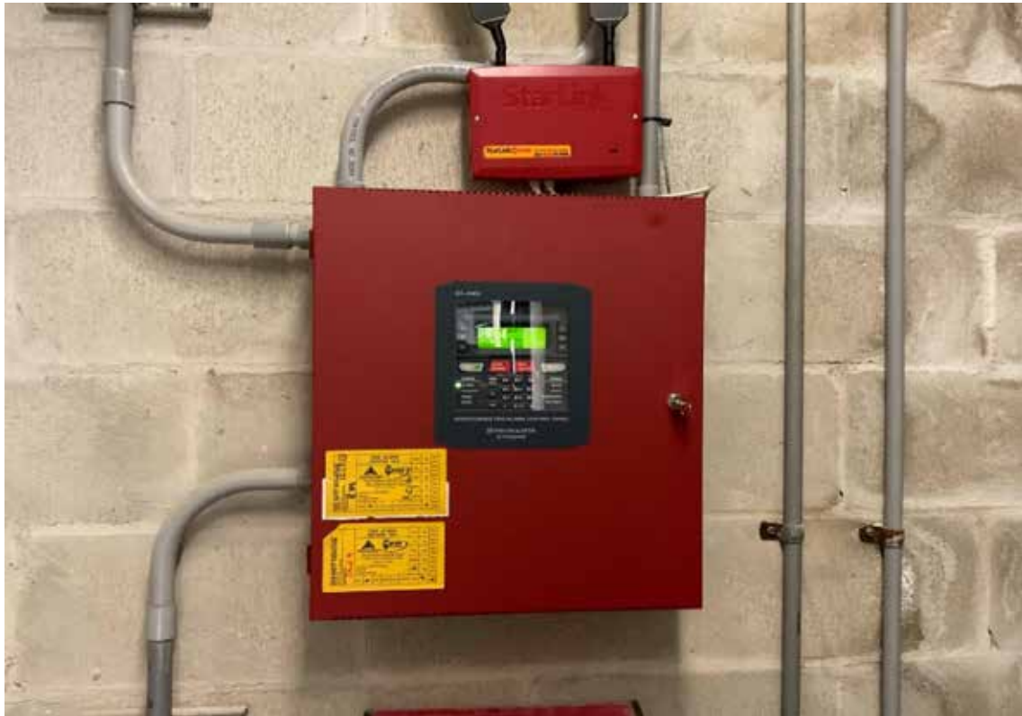
Bldg 300 - Fire Alarm Panel
