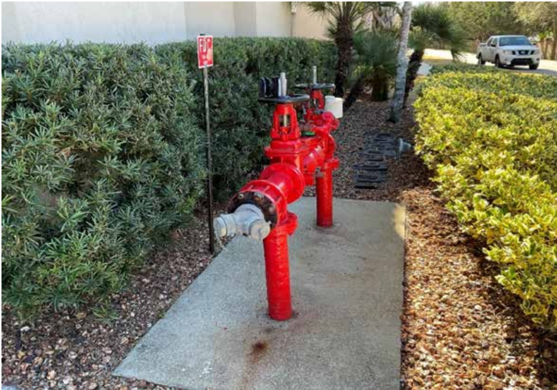
Bldg 100 - Backflow Preventer
