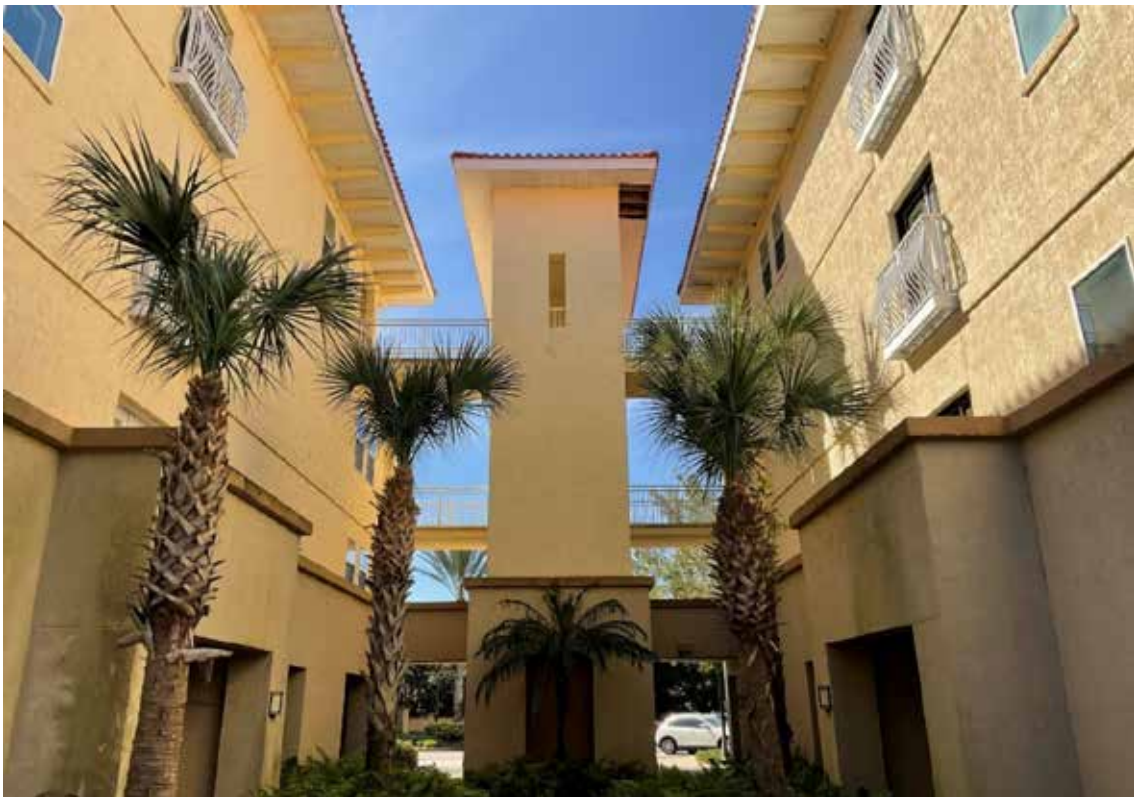
Bldg 200 - Missing Soffit
