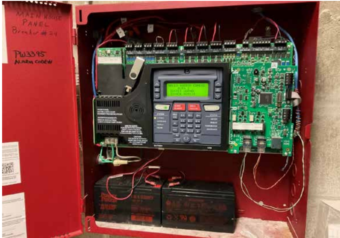
Bldg 200 - Fire Alarm Panel
