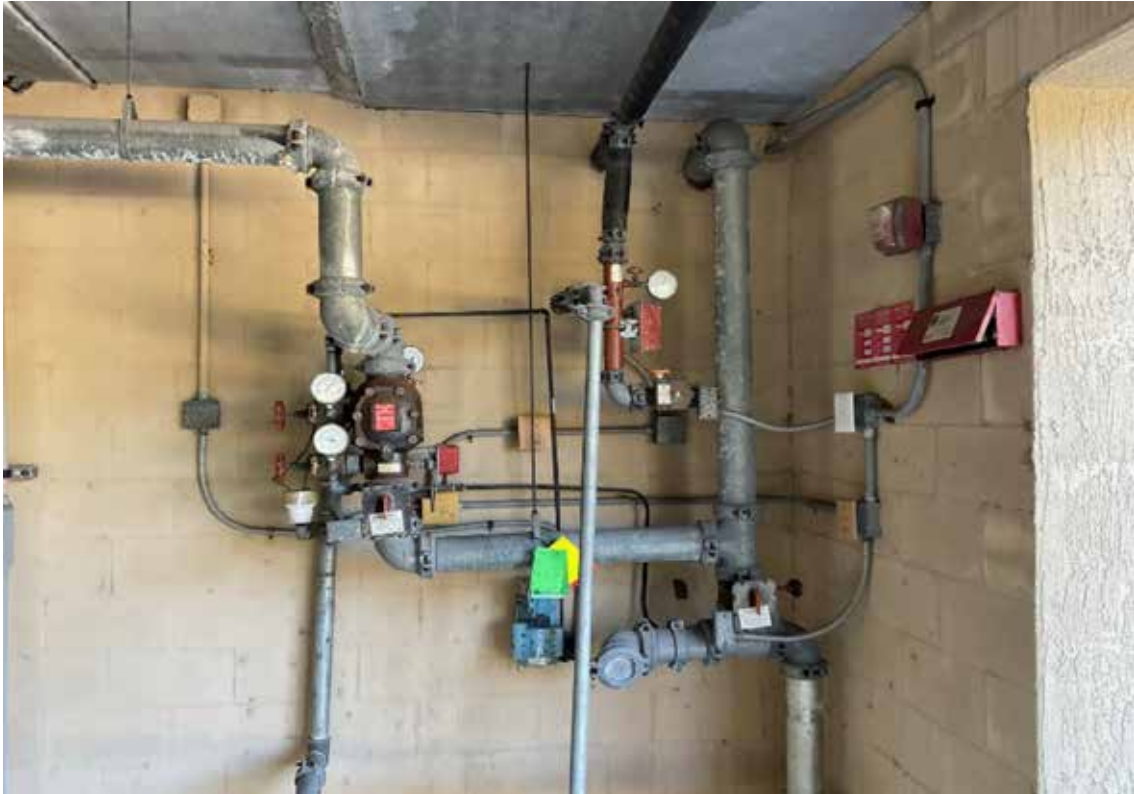
Bldg 100 - Dry Fire System
