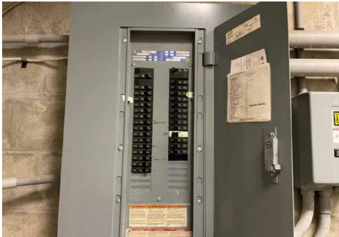
Bldg 200 - Electrical Breakers
