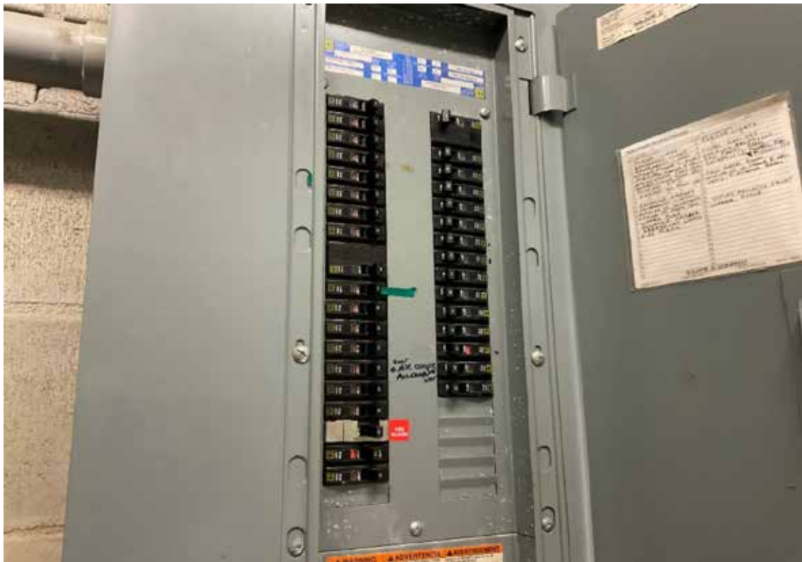
Bldg 300 - Electrical Breakers
