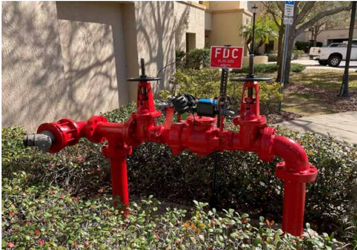
Bldg 200 - Backflow Preventer
