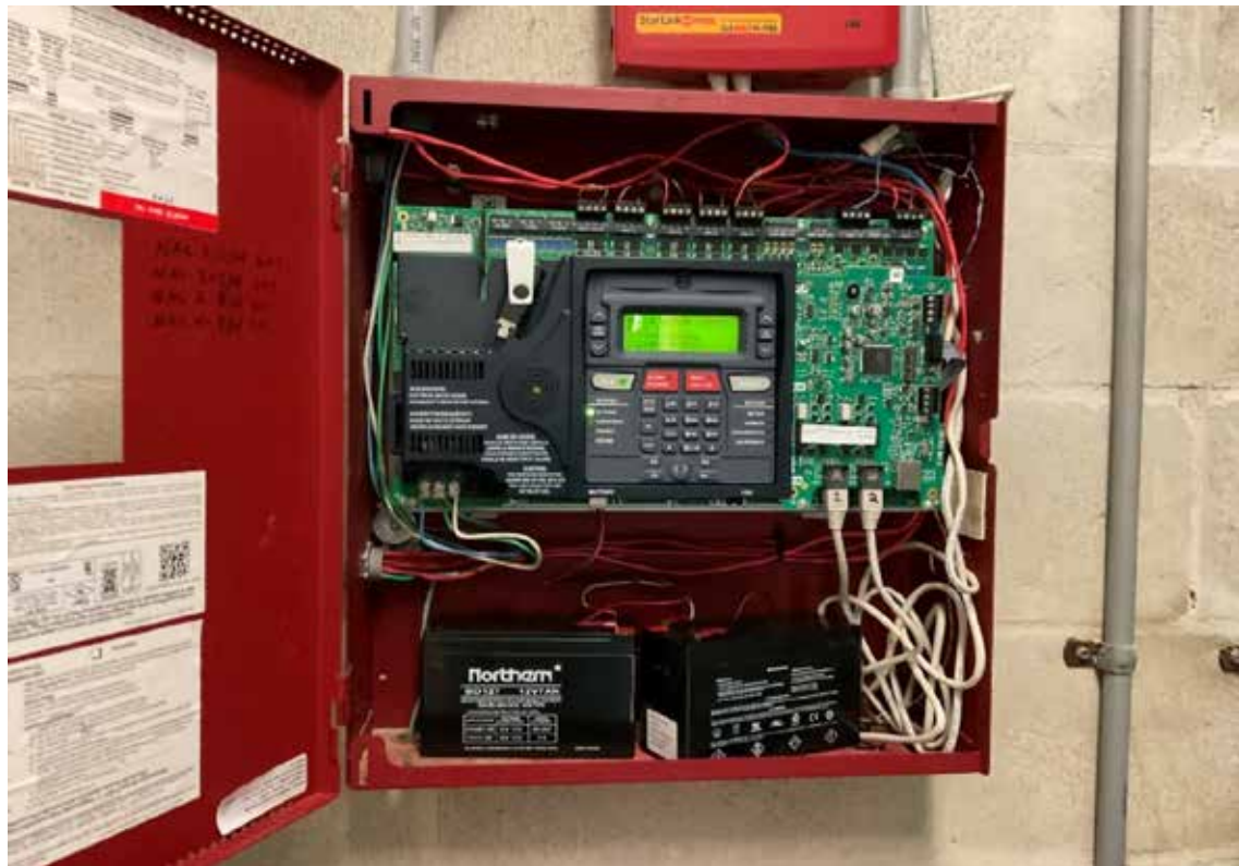
Bldg 300 - Fire Alarm Panel
