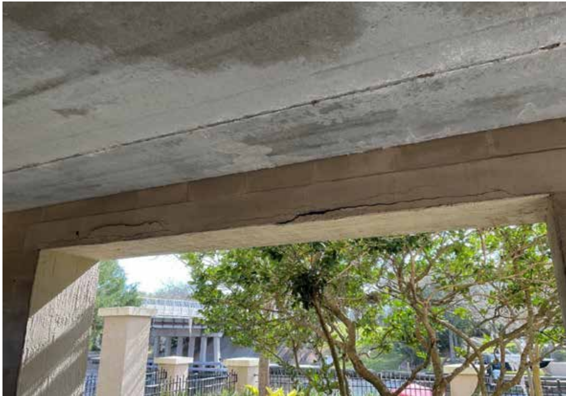
Bldg 300 - Spalling Concrete
