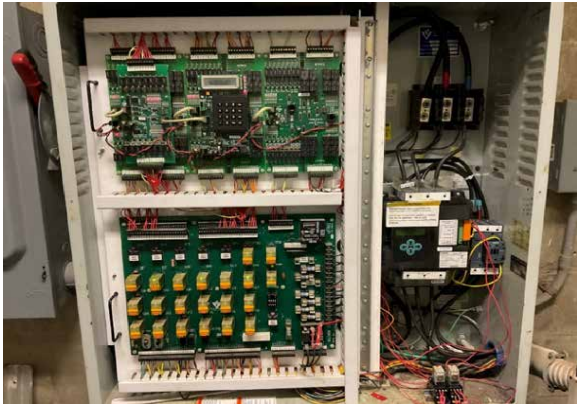
Bldg 200 - Elevator Equipment
