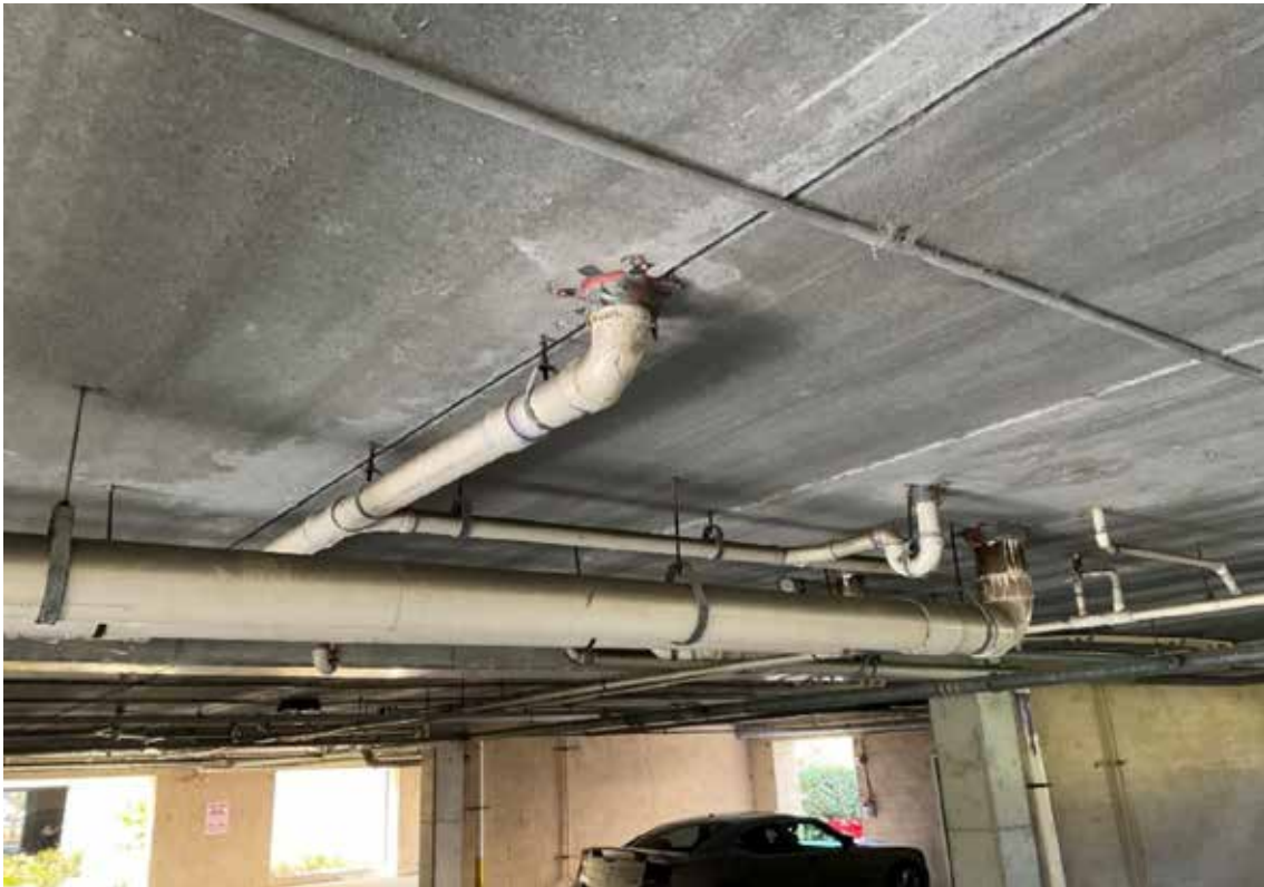
Bldg 300 - Plumbing Lines
