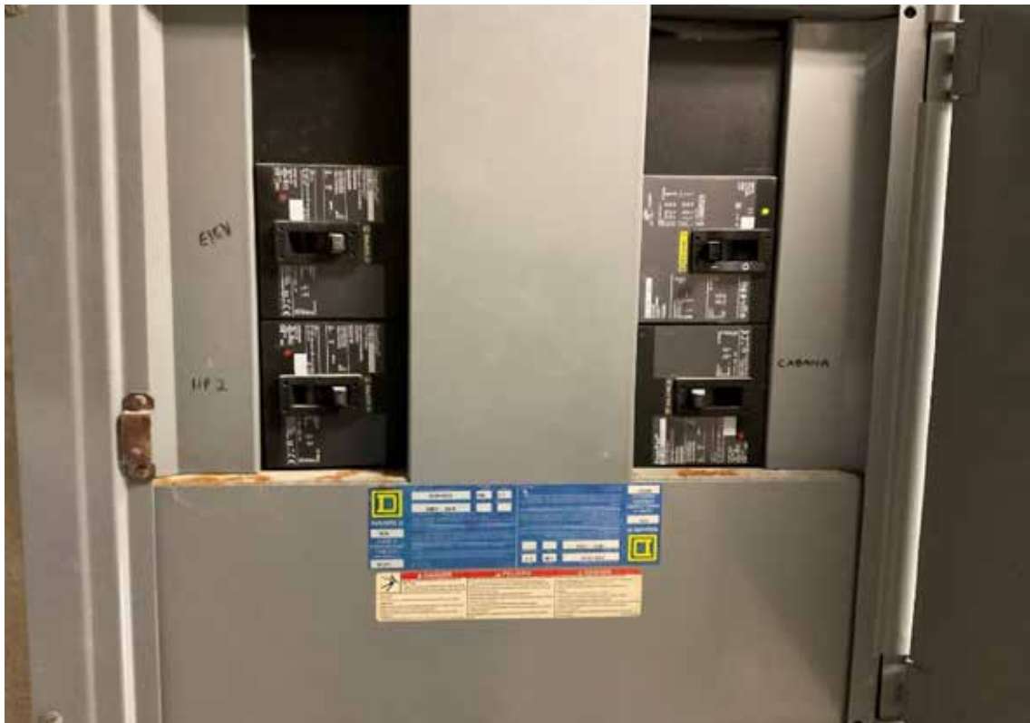
Bldg 100 - Electrical Breakers
