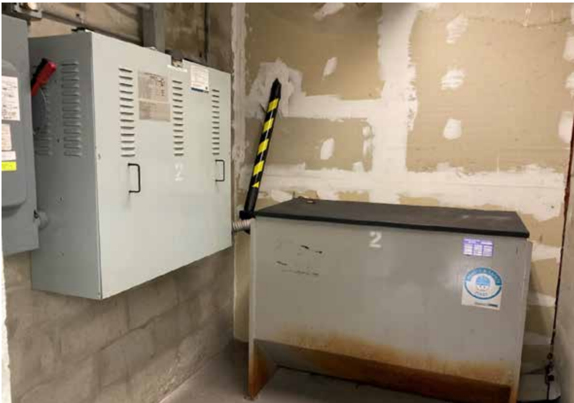
Bldg 200 - Elevator Equipment
