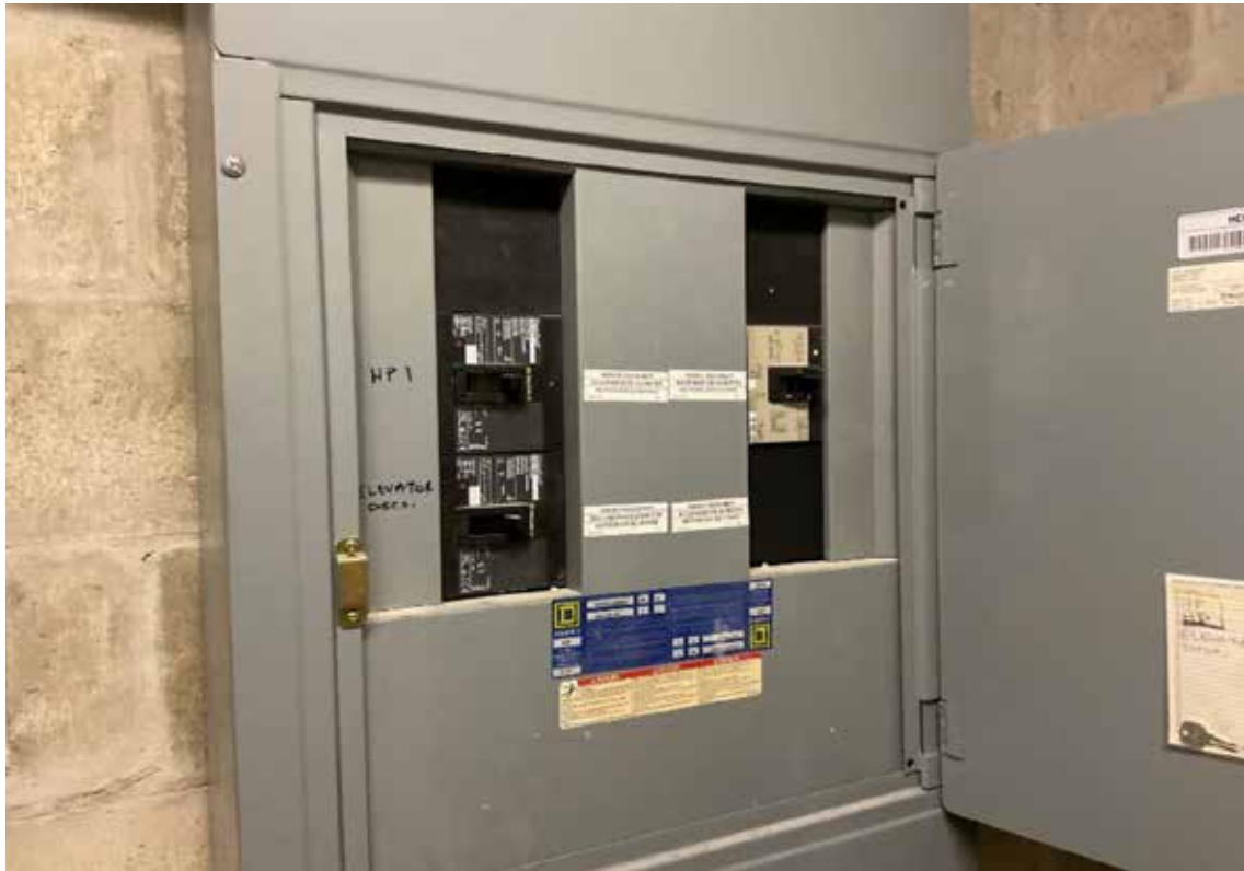
Bldg 200 - Electrical Breakers
