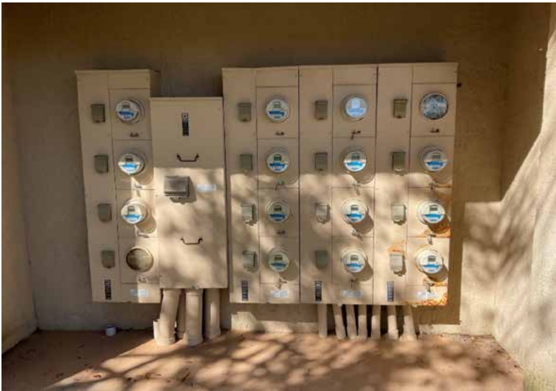
Bldg 200 - Electrical Panel/Meters
