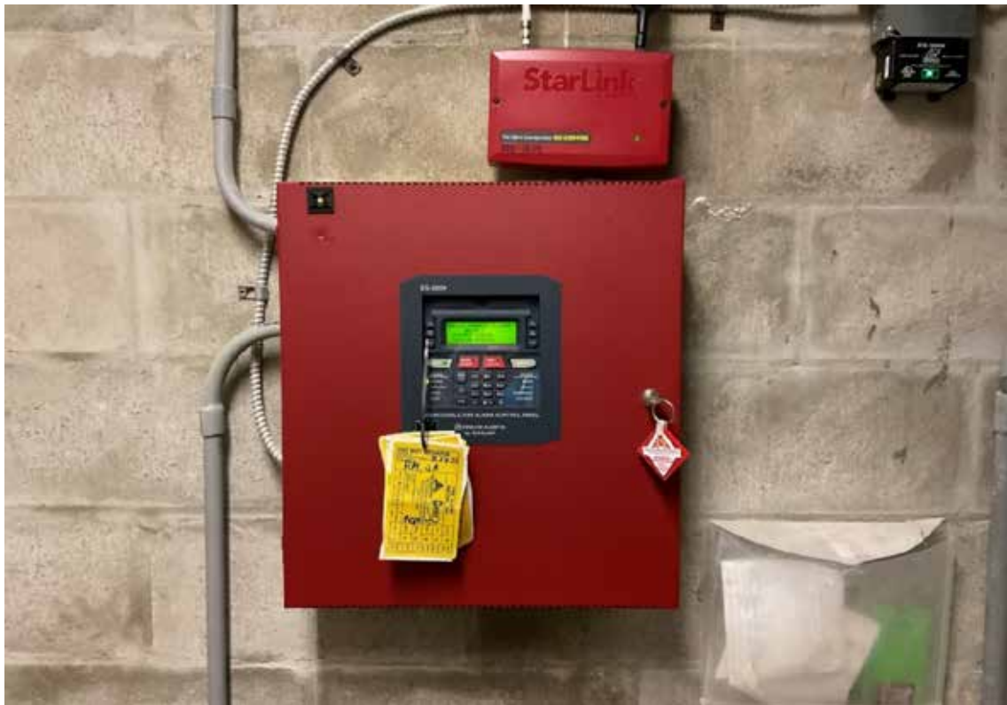
Bldg 200 - Fire Alarm Panel
