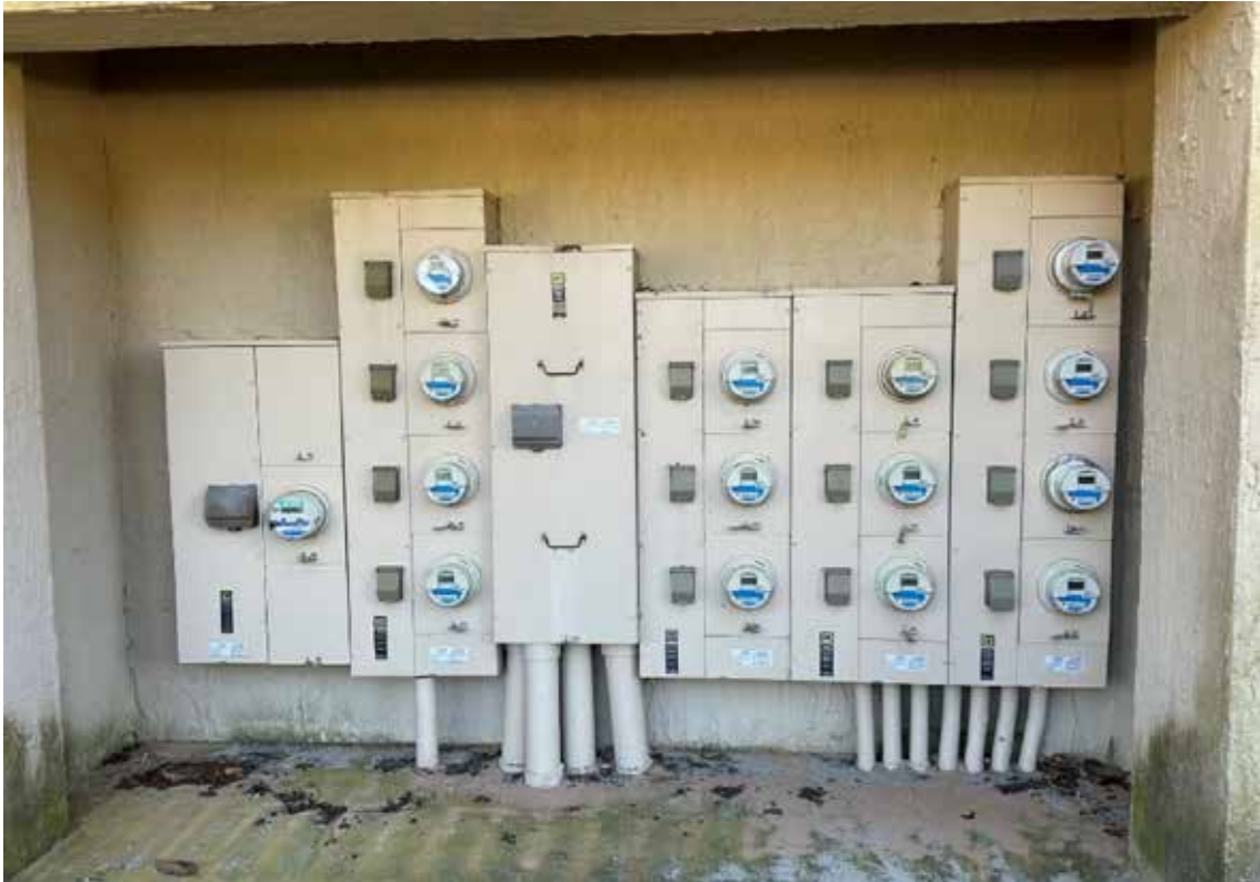
Bldg 100 - Electrical Panel/Meters
