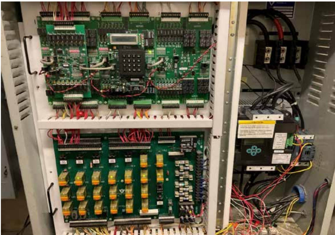
Bldg 300 - Elevator Equipment
