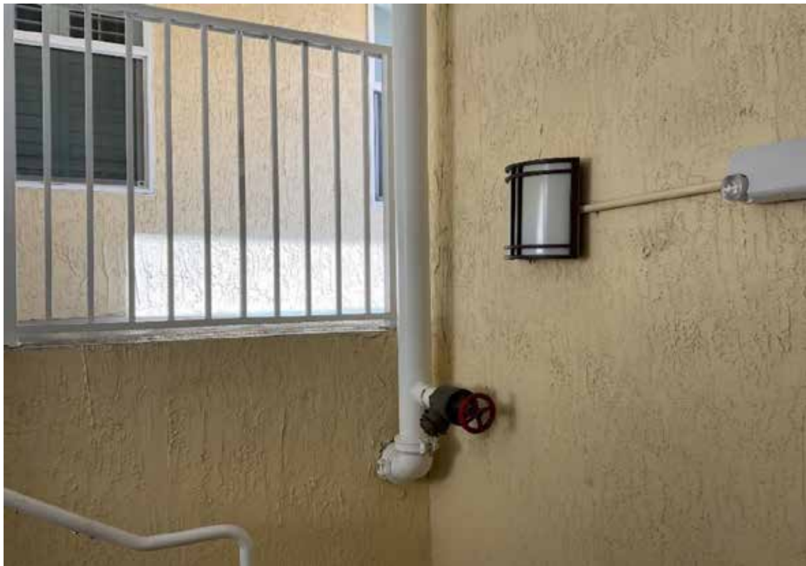
Bldg 200 - Fire Standpipe
