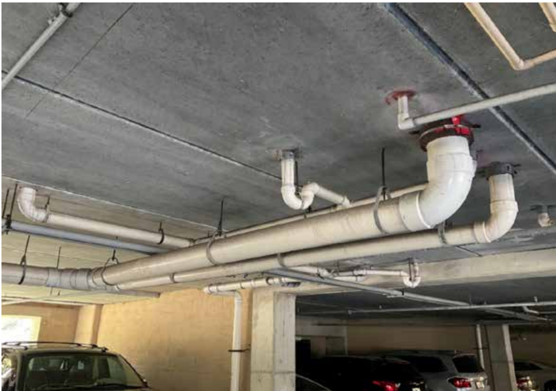
Bldg 100 - Plumbing Lines
