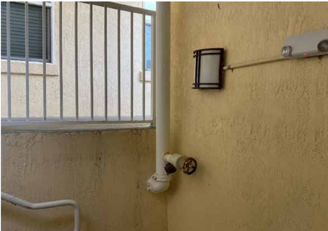
Bldg 300 - Fire Standpipe
